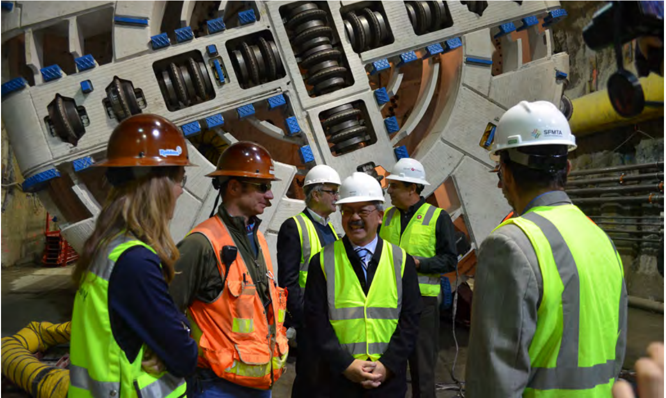
Mayor Lee tours construction of Central Subway, which will better connect communities
